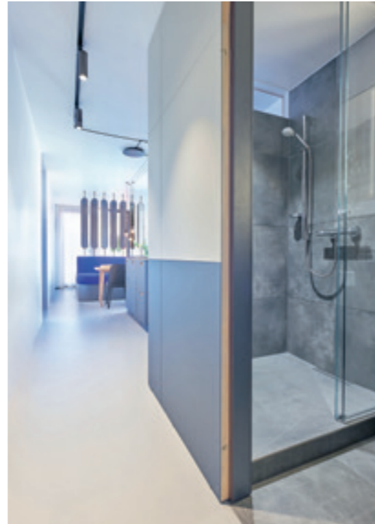
↑ Despite its modest size of 3 m 2 , the bathroom in the smaller container impresses thanks to its exceptional level of comfort. This is in no small part down to the shower with the Geberit CleanLine shower channel.
